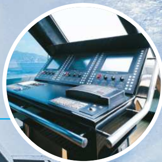
Inside the control room
