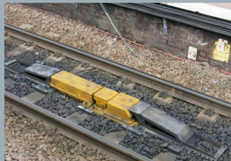
Automatic warning systems can also alert people working on the tracks further down the line of an oncoming train
