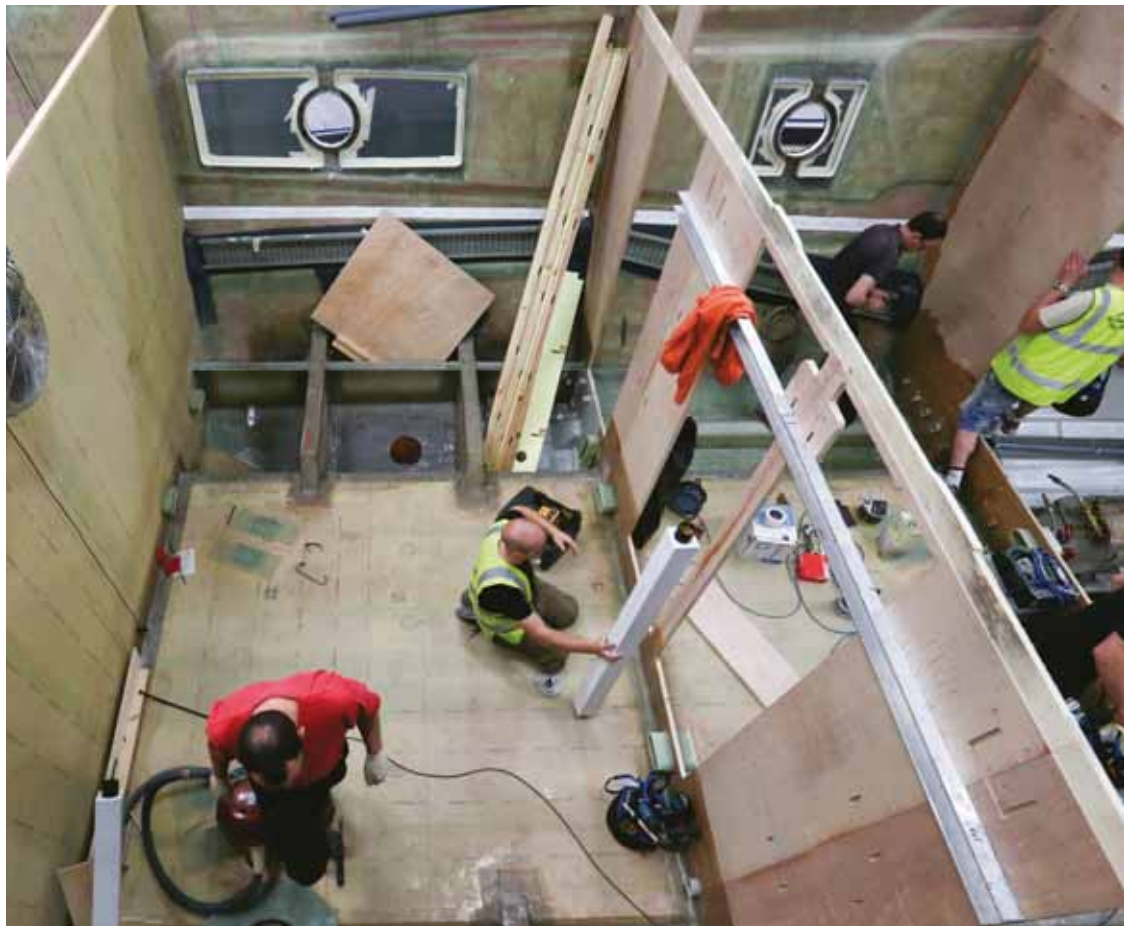
Below: Individual rooms are laid out by carpenters, electricians, mechanics, plumbers and engineers all working together across the yacht
