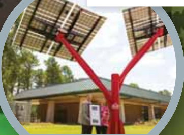
The solar-powered charging station on The Ray opened in October 2015 and was the first of its kind in Georgia
