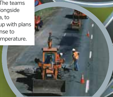
Data from the project can help the team adapt to the challenges of a changing climate, thereby helping them to improve highways
