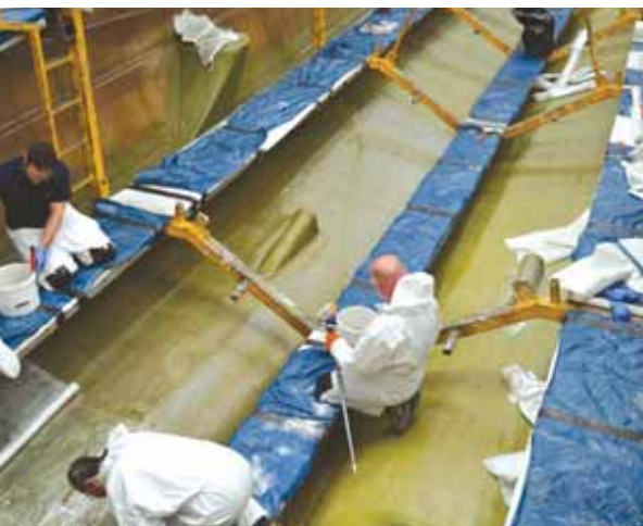
A team coats the inside of the hull's mould with fibreglass during the first stages of construction
