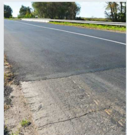
You may notice the difference in noise level when driving between old and new road surfaces
